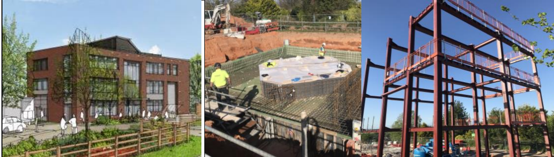
Figure 8: Vsimulstors @Exeter building (left), inertia block, and building frame (right).
