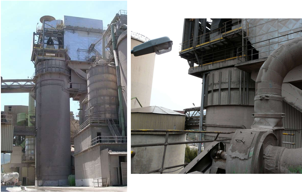
Figure 9. Completed dedusting installation on top of an existing silo. General view (left) and support platform (right). Photos taken in 2011.
