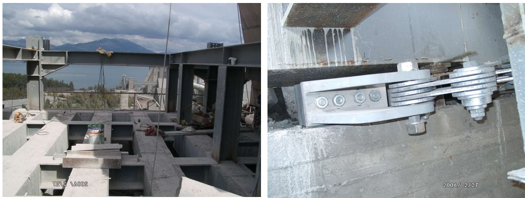
Figure 7. Dedusting installation on top of an existing silo. General view of rigid platform (left) and detail of friction damper (right).
