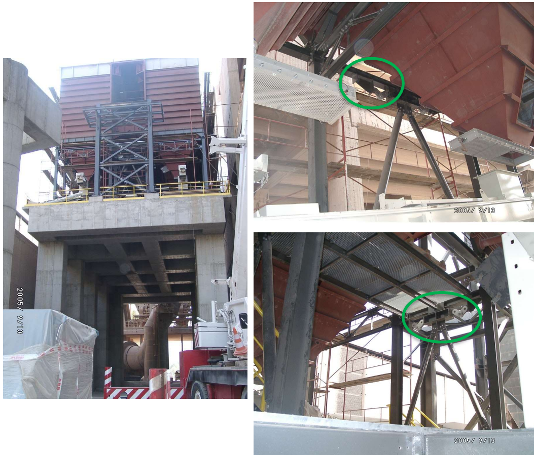
Figure 10. Installation of heavy filter with geometrical constraints. General view (left) and braces with dampers (right).
