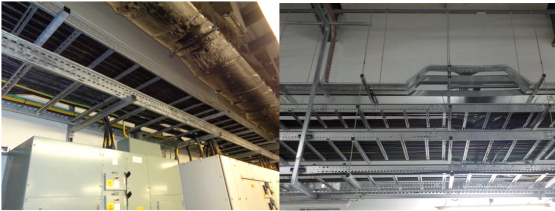
Figure 6. Examples of heavily loaded cable trays designed as secondary systems.
