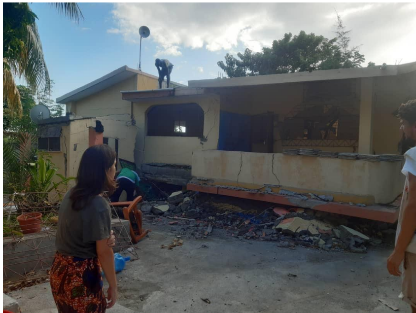
Figure 2. Collapsed MSF guesthouse in Port-à-Piment, image courtesy of MSF.
