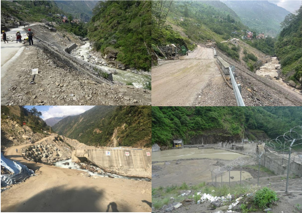
Figure 10. The recovery of road and hydropower infrastructure along the Ariniko highway, left 2017, right 2022.
