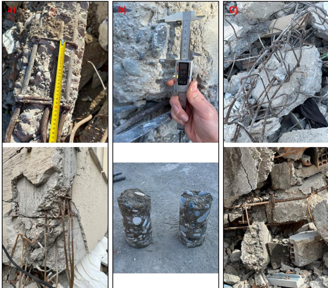
Figure 5. Typical material and detailing deficiencies in pre-2000 buildings; a) Smooth-surfaced rebars with 90° hooks at the ends of stirrups and deficient detailing; b) Anomalous size and shape of aggregates; c) Excessive corrosion and poor reinforcement detailing.
