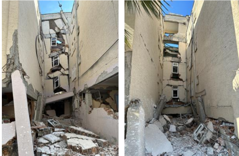
Figure 9. Failures of two identical buildings.
