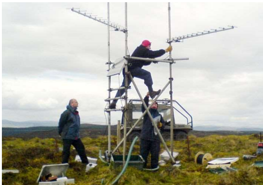
Figure 1- FM radio re-transmission station being repaired after high winds blew an aerial out of position.
