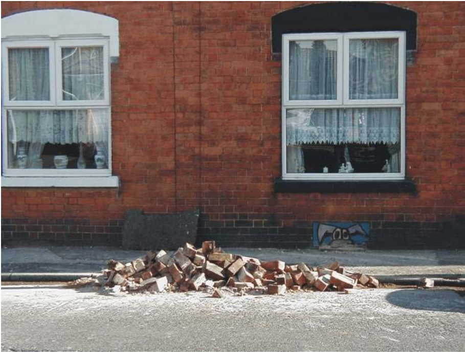
Figure 2. Damage to a chimney in the Bloxwich area from the Dudley Earthquake
